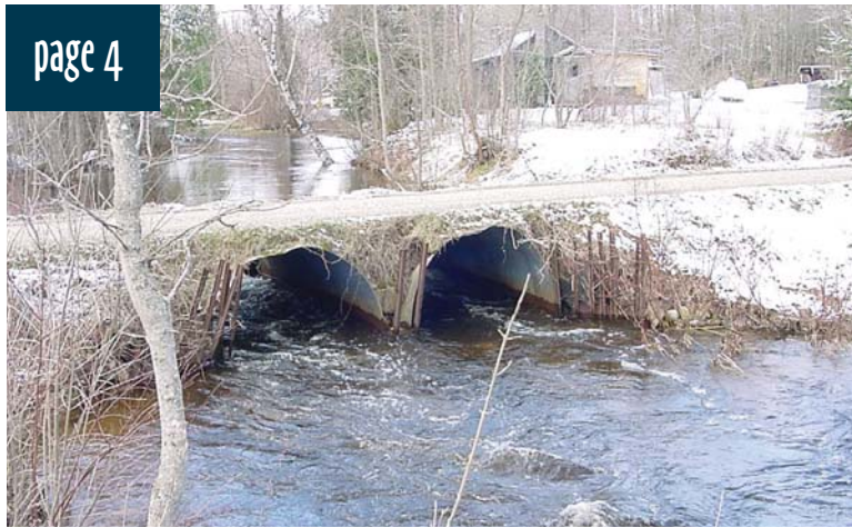
Problematic culverts on the Carp River.
